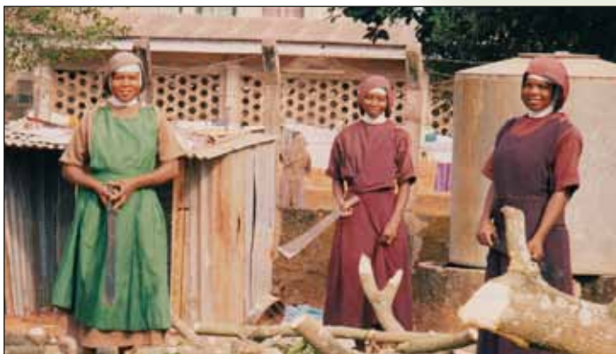
Clearing a space for the building of a new poultry house at St. Scholastica Benedictine Abbey
